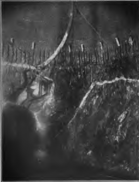
PLATE 3. SHOWING GROUT HOSE CONNECTED UP TO PIPE READY FOR GROUTING A SMALL STREAM, ABOUT 5 GALLONS PER MINUTE, NOT SHUT OFF BY ORIGINAL GROUTING. ABOVE ARE SHOWN ORIGINAL GROUT PIPES, NOW CUT OFF TO ALLOW THE SHAFT TO BE DRILLED. MARKS OF THE HOLES PUT DOWN TO TAKE OUT THE FIRST ROCK CUTS ARE ALSO CLEARLY SHOWN ON THIS PLATE AND, PLATE 2.
